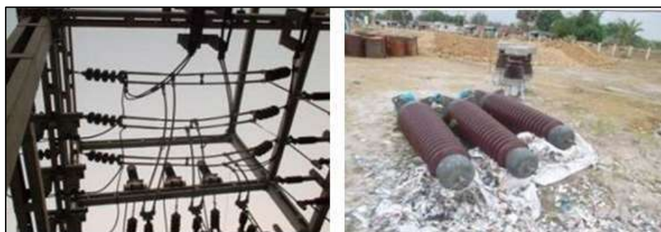
Figure 3.3: Disc insulators for transmission line
