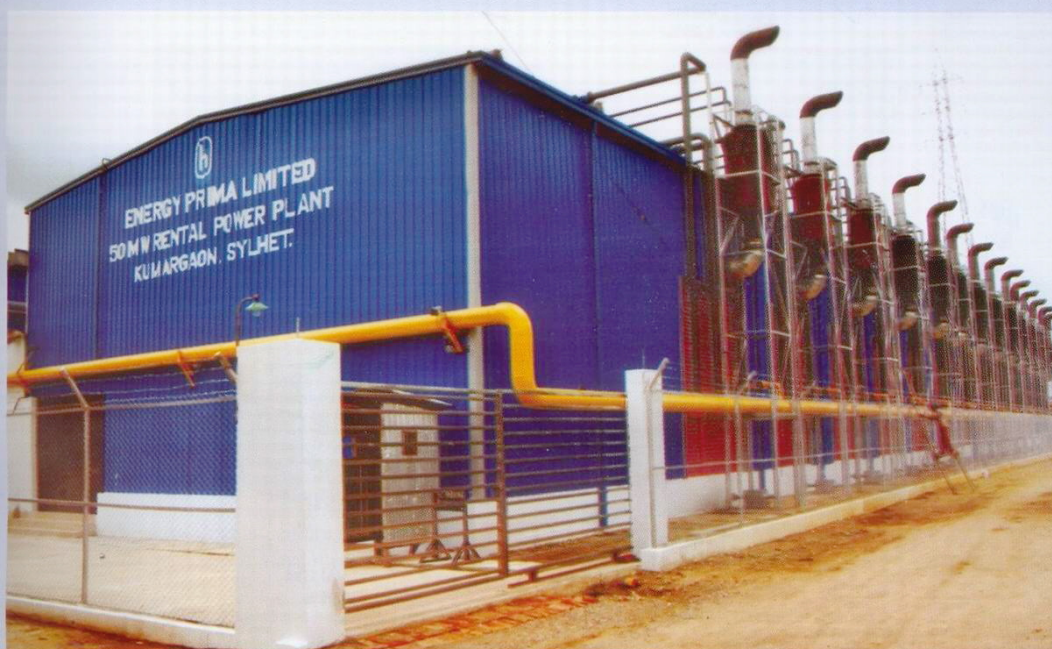
Newly constructed Kumargaon (Sylhet) 50 MW Rental Power Plant.
