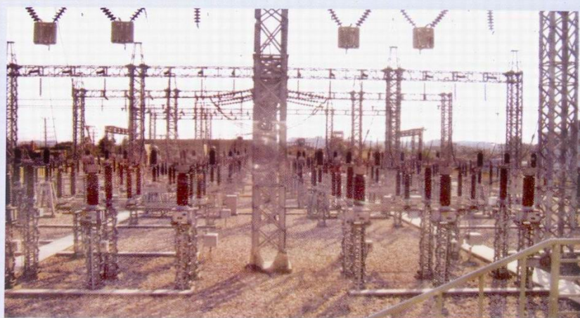
Bakalia 132/33 KV Grid Sub-station constructed under Greater Chittagong Power Distribution Project.
