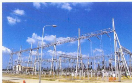
Aminbazar 230/132 kV Sub-station
