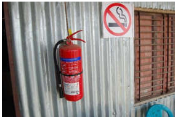
Fire extinguisher at Site office
