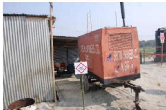
DG Set at construction site
