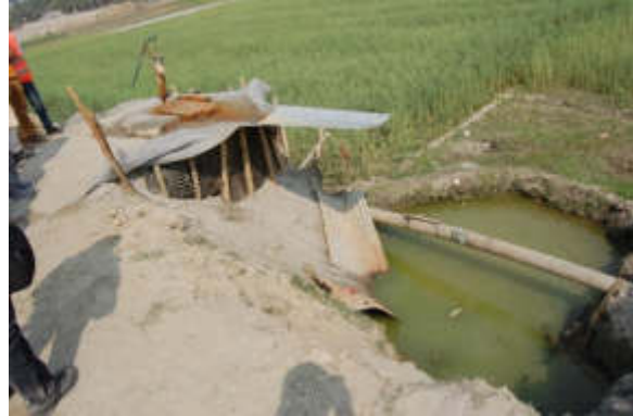
Tube well and Grey water storage pit
