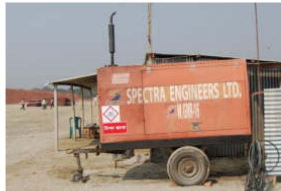
Safety precaution signage at DG set
