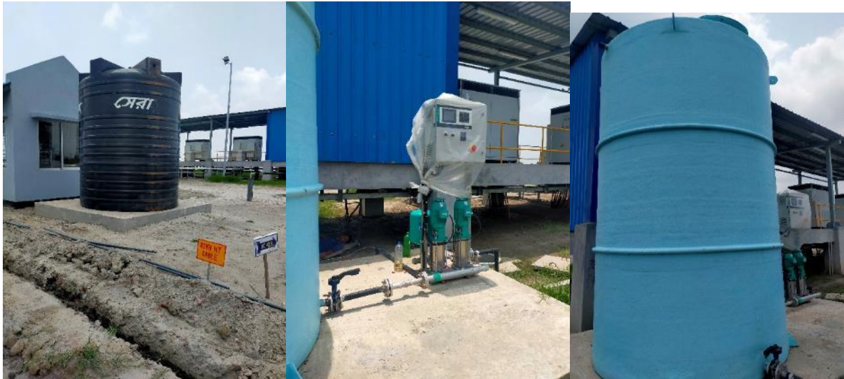
Photo 4: Water Reserve Tanks
