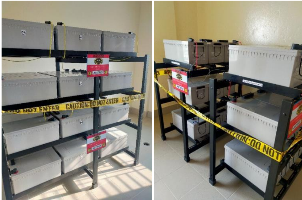
Photo 6: 20 KVA Battery backup
