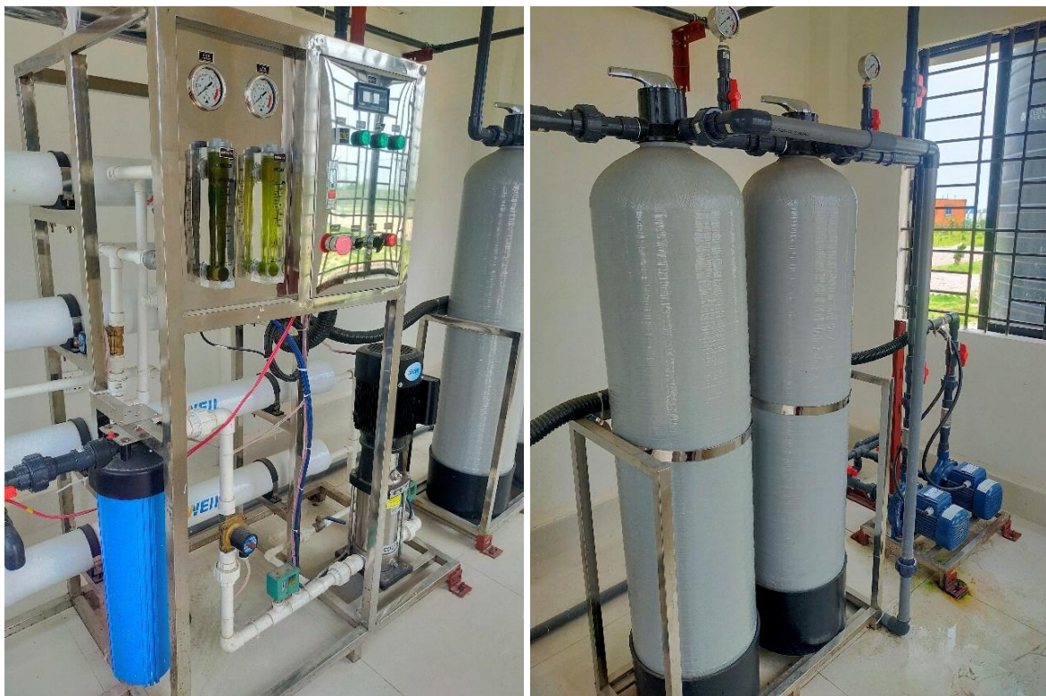
Photo 3: RO System for groundwater treatment
