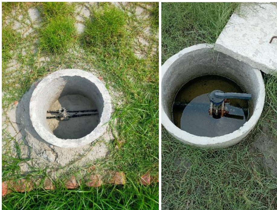
Photo 5: Water Valves for Module Cleaning
