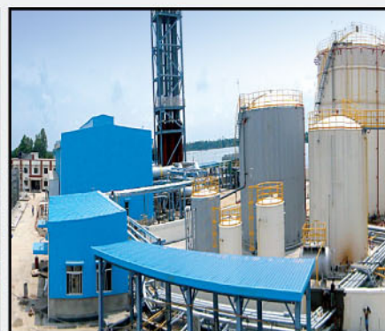
Baghabari 50 MW Peaking Power Plant
