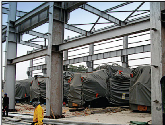
Katakali 50 MW Peaking Power Plant Expected Commissioning Date : April 2012
