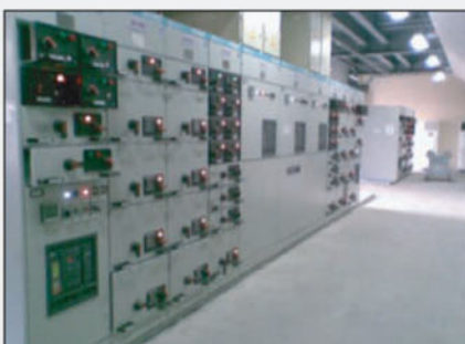
Baghabari 50 MW Peaking Power Plant
