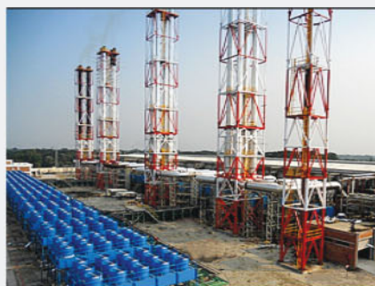
Gopalganj 100 MW Peaking Power Plant
