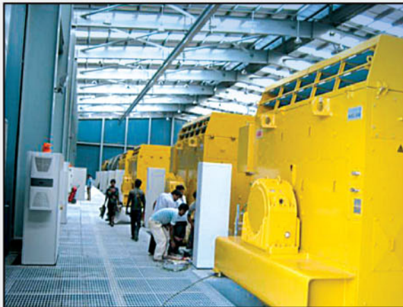
Keraniganj (Power Pack) 100 MW Quick Rental Power Plant Expected Commissioning Date : February 2012
