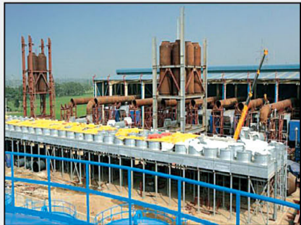
Julda, Karnophuli (Acron) 100 MW Quick Rental Power Plant Expected Commissioning Date : February 2012
