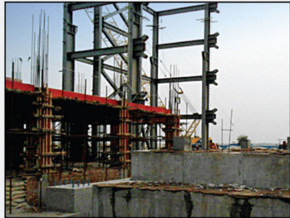
Sirajganj 150 MW Power Plant Expected Commissioning Date : July 2012
