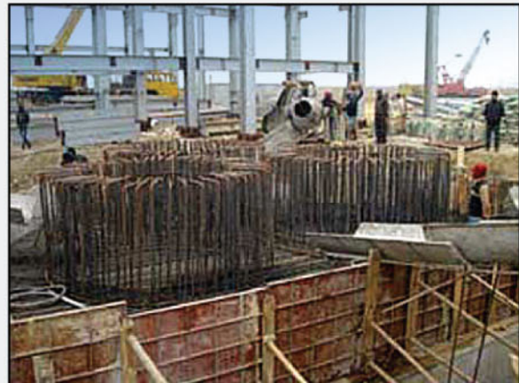
Shantahar 50 MW Peaking Power Plant Expected Commissioning Date : March 2012
