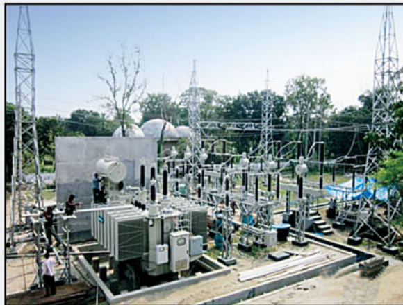
Katakhali, Rajshahi (NPSL) 50 MW Quick Rental Power Plant Expected Commissioning Date : February 2012
