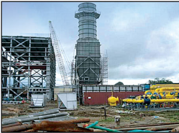
Sylhet 150 MW Power Plant Expected Commissioning Date : February 2012
